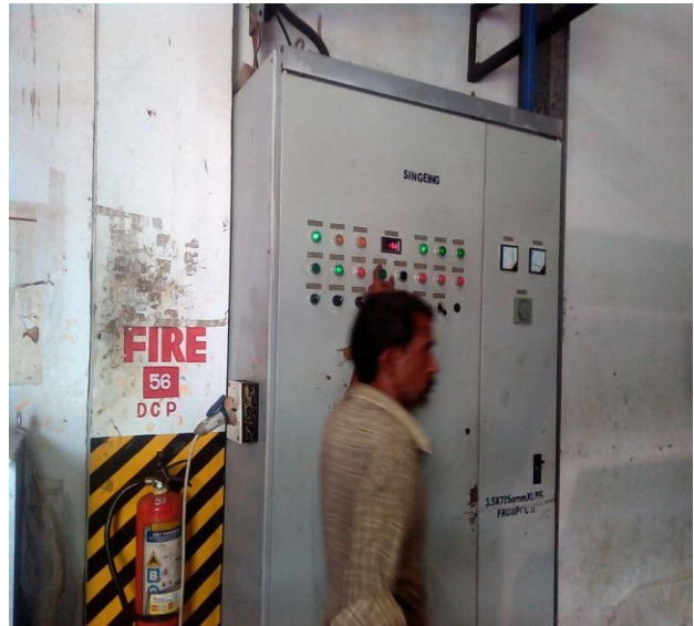
switch on the power panel
