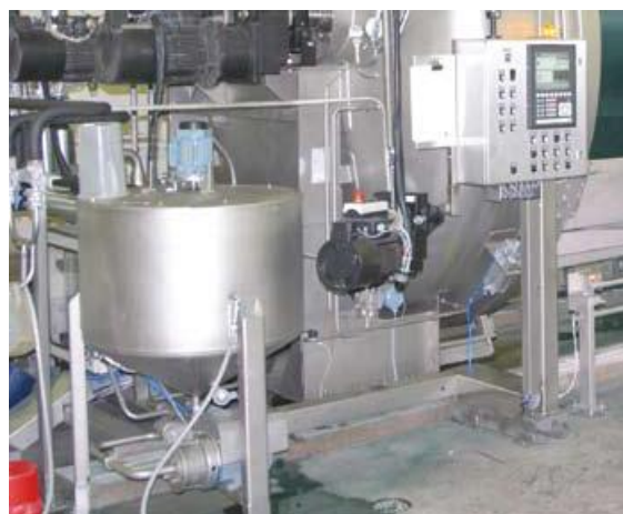
Preparation tank & main panel
